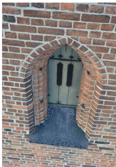
Fig 25: Revleluge – gitter mangler
