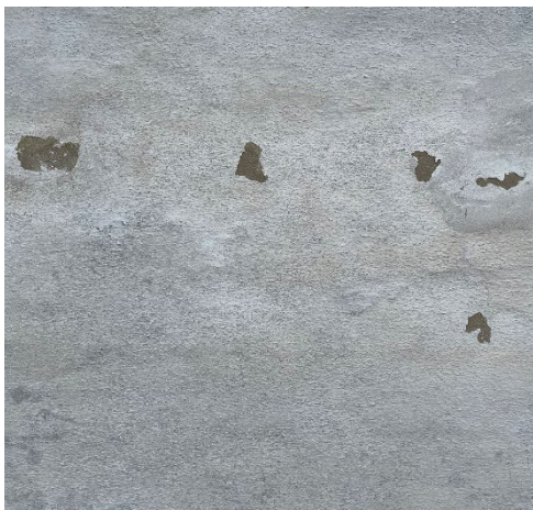
Figur 6. Afskalning over cementpuds.
